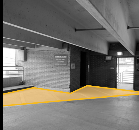
Blocked space before stair/elevator
